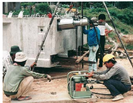
Fig. 18: TENSAM 1700 kN stressing jack and mini pump unit – post-tensioned beams on a construction site in Malaysia
